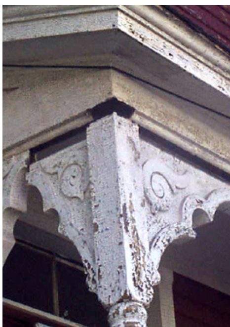
FIGURE 1.2 Deteriorated residential paint on house trim.
