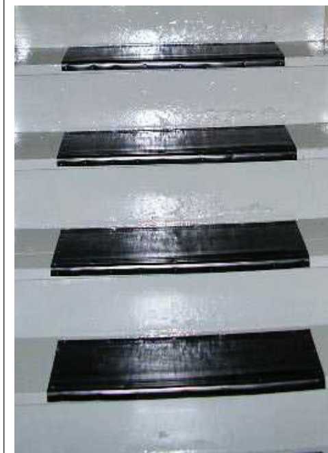
FIGURE 5.6b Friction hazard on stairs post-treatment.
