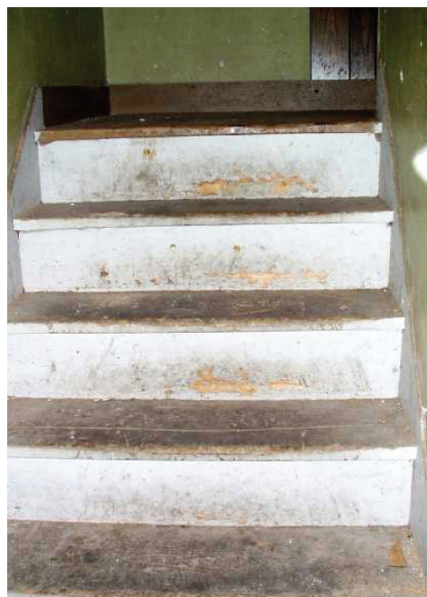
FIGURE 5.6a Friction hazard on stairs pre-treatment.
