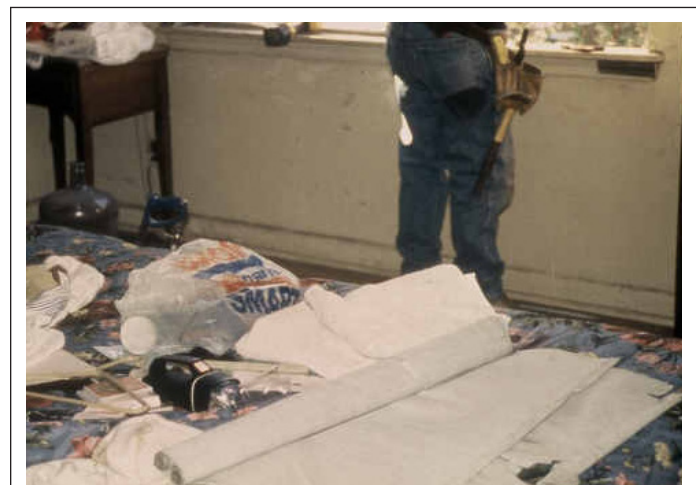
FIGURE 4.3 This worksite was not properly prepared for lead-disturbing work by removing the occupant's belongings.
